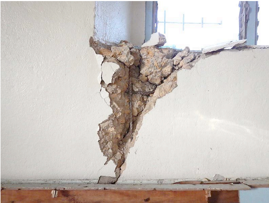
Figure 24. Close-up view showing steel reinforcing bars exposed by spalled concrete. These are twisted bars, which is a type common in the early 20th century. From spall locations like this it is clear that the concrete mix uses aggregate larger than recommended today, and that there are very few horizontal reinforcing bars.
