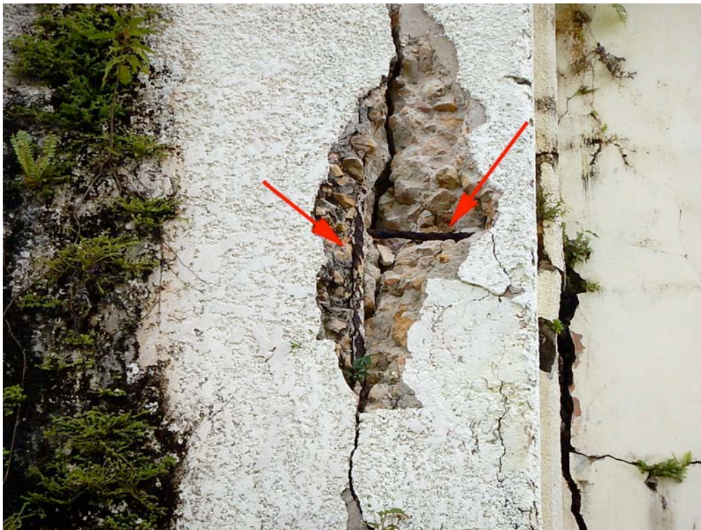
Figure 50. Detailed view of the crack at the southwest corner, showing exposed twisted reinforcing bars, and also exposed concrete with reveals large aggregate.
