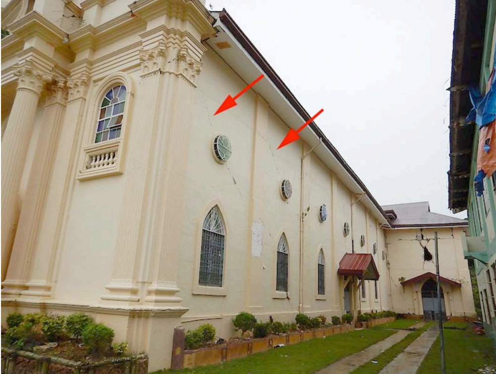
Figure 13. View of the southwest corner, and nave south side elevation and south transept, showing typical diagonal cracks at the arrows. See also fig. 28 for the interior view of the same cracks. The transept wall beyond is severely cracked, with horizontal cracks at a cold joint, and vertical cracks at the reentrant corner with the nave wall. The transept walls sustained more damage from the earthquake than the nave walls.
