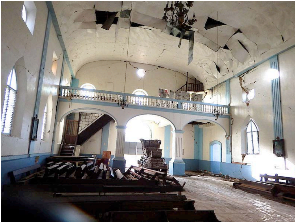
Figure 20. View of interior looking west towards the choir loft. Note the vertical and diagonal cracks on all the walls and the falling sheet metal ceiling.
