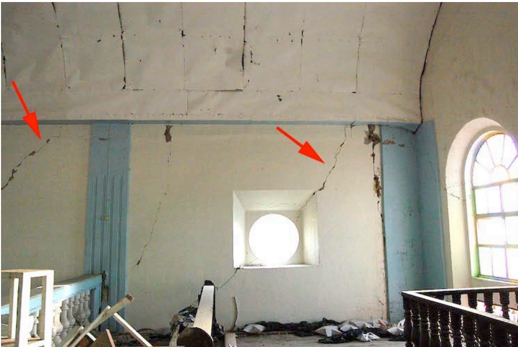
Figure 28. View of the southwest corner at the balcony level. The diagonal cracks at the arrows are the same exterior cracks shown in fig. 13. Note also a vertical crack at the left of the blue pilaster. All of the cracks appear to be the result of movement of the building and front facade to the west, and a possibly overturning of the front facade.
