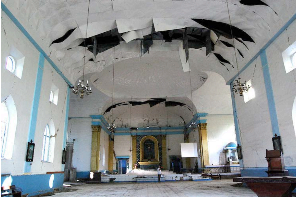
Figure 19. View of the church interior looking towards the altar. Note the vertical and diagonal cracks on all the walls and the falling sheet metal ceiling.
