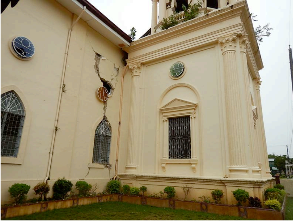
Figure 15. View of the corner where the bell tower is attached to the north nave wall. The cracking in the nave wall above the openings appears to have been caused by rocking of the bell tower and subsequent pounding.
