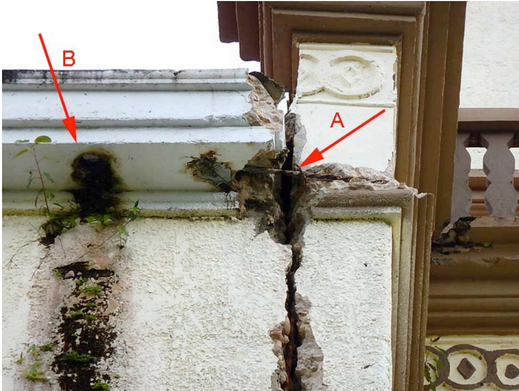
Figure 49. Detailed view of the crack at the southwest corner. Note the reinforcing bar at “A,” which appears to be for the cornice. At “B” is a gutter outlet, which is missing its downspout, and has caused extensive plant growth on the wall and in cracks in the wall.
