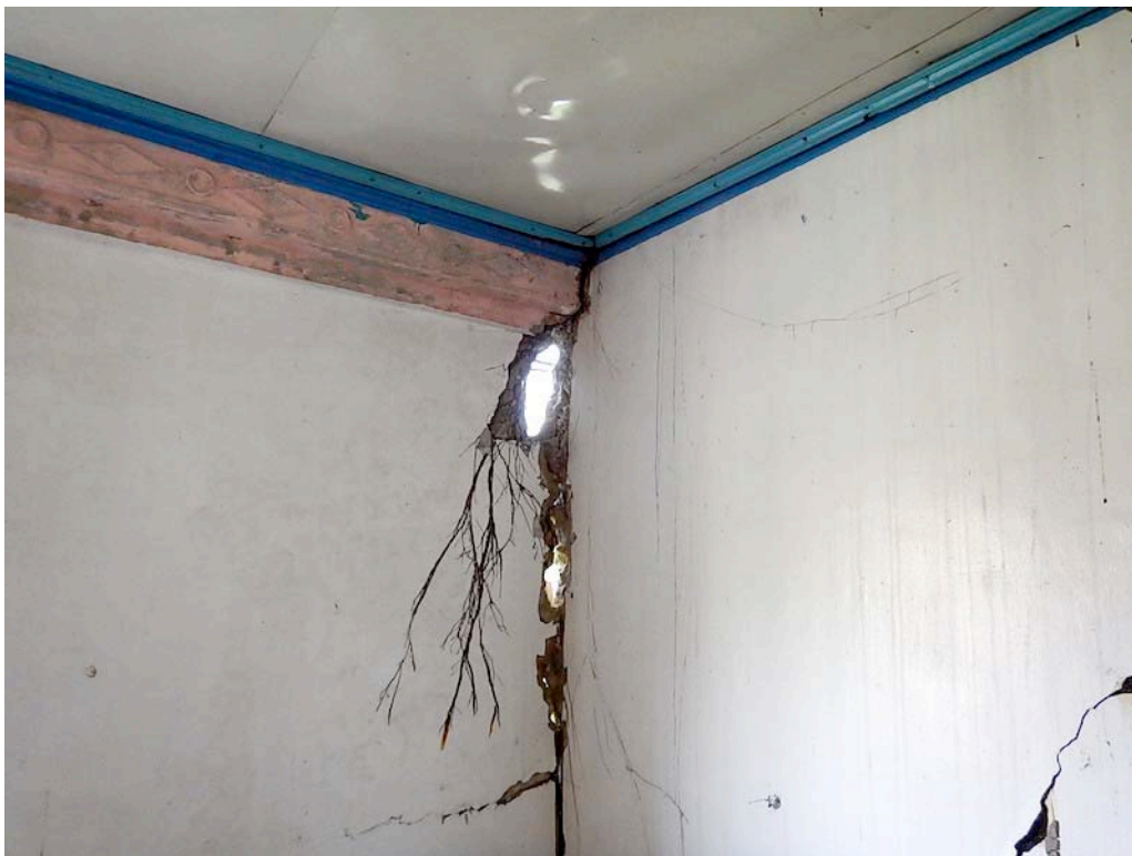
Figure 58. Close-up view of the southeast corner crack from the interior. Compare with fig. 46. At this location it can be seen that the reinforcing bars are of small size and inadequately spaced. Note also plant roots from plants growing on the exterior.
