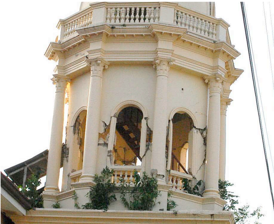
Figure 14. View of the bell tower cupola, exhibiting severe cracks of its hexagonal walls from rocking and possible twisting. Plant growth is abundant around the cupola. See fig. 22 for underside.
