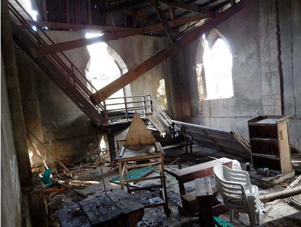
Figure 27. View of the southeast corner room, with collapsed roof structure, and cracked and displaced sections of concrete wall. See exterior view in fig. 17.
