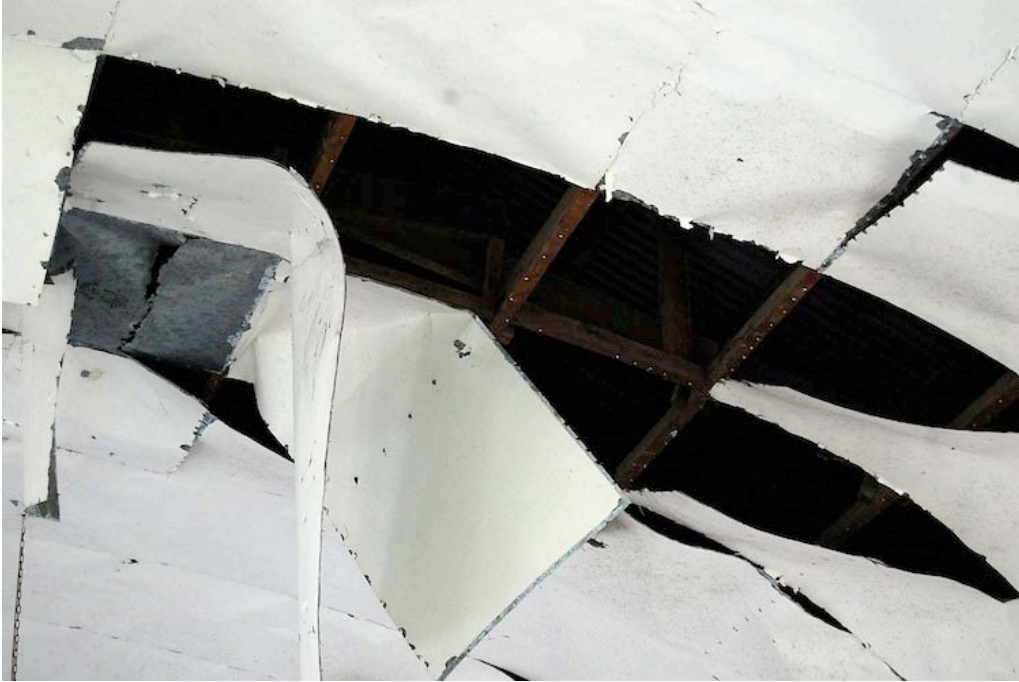
Figure 21. Close-up view of the ceiling area with exposed wood framing and falling sheet metal. Note that there are two layers of sheet metal ceiling and that the sheet metal has pulled through the fastener holes.
