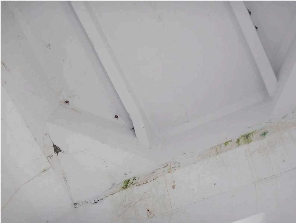
Figure 22. Underside of bell tower ceiling, showing that the construction is modern, with diagonals at the corners to resist twisting of the structure during an earthquake. Note the green stains from biological growth at leaks in the roof above.
