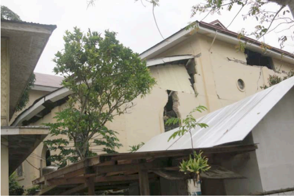
Figure 17. View of the southeast corner, where the roof has collapsed. See interior view in fig. 27.
