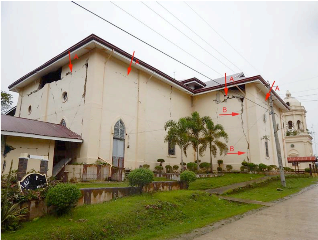
Figure 16. View of the northeast corner and north transept. The horizontal crack at “A” appears to be a cold joint boundary between two phases of construction. The vertical crack at “B” is likely due to overturning of the north transept wall.
