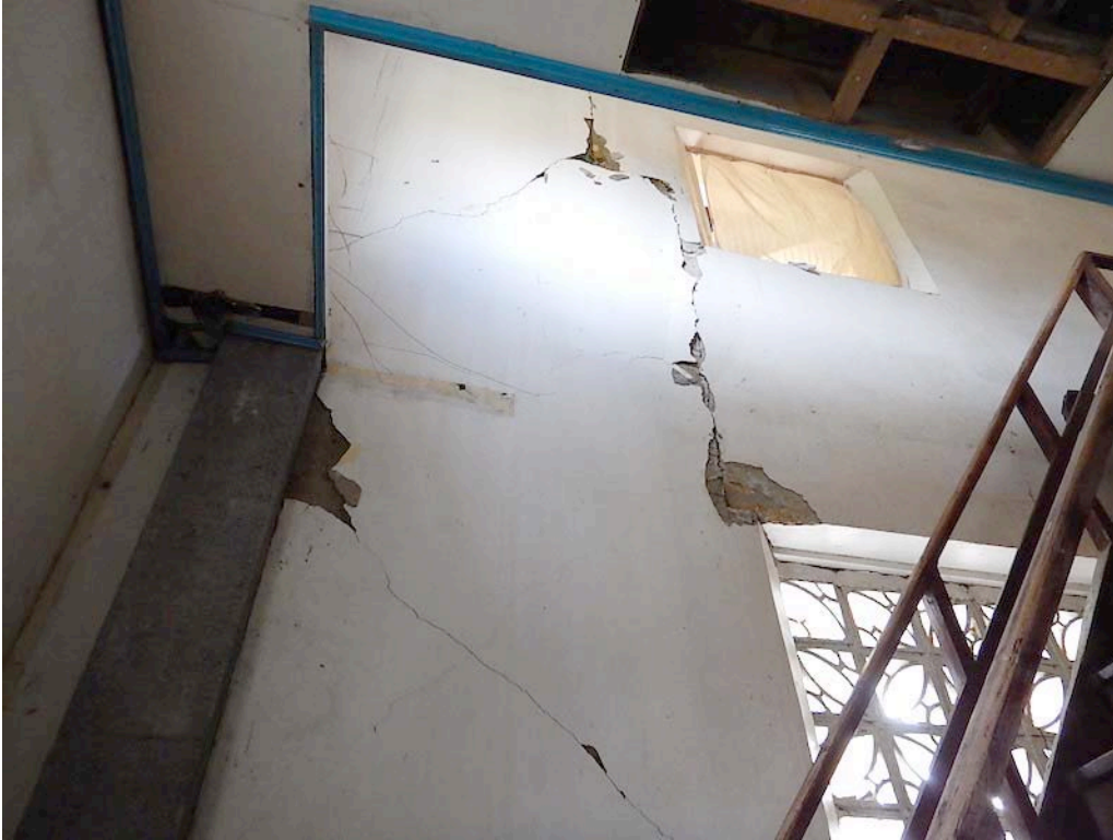
Figure 59. View of the inside face of the front facade at the choir loft. The vertical cracks appear to be at the boundary between construction phases, and extend through the exterior.
