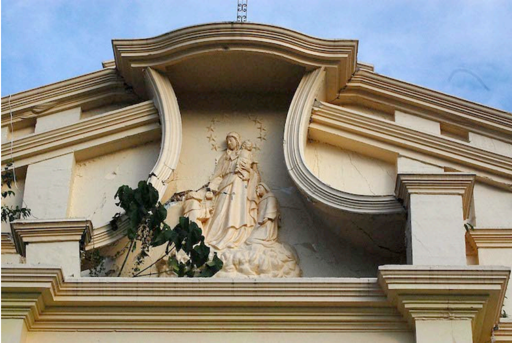
Figure 11. View of the highly articulated pediment over the front facade, exhibiting numerous cracks in all directions, probably from rocking motion. Plant growth in the pediment is a sign of the presence of moisture and soil.
