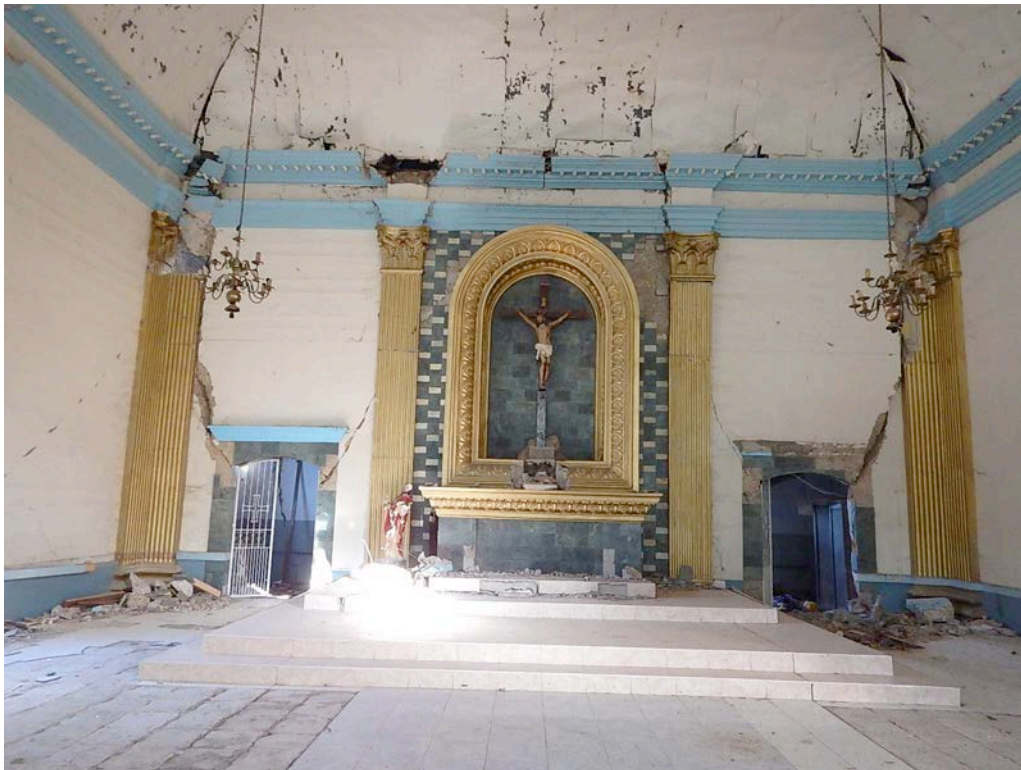
Figure 26. View of the altar wall, with diagonal cracks passing through the door openings.
