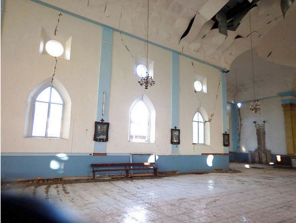
Figure 23. View of the north nave wall, showing pervasive vertical and diagonal cracks passing through the windows, which are a discontinuity in the wall.
