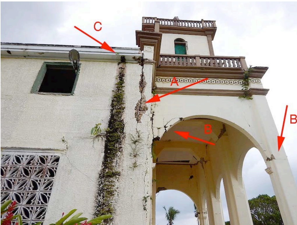
Figure 48. Detail of figure above, showing at "A" vertical crack and hinge cracks at "B," both from rocking of the portico. At "C" is a gutter outlet, which is missing its downspout, and significant plant growth from excessive water saturation of the concrete. See details in the following figures.
