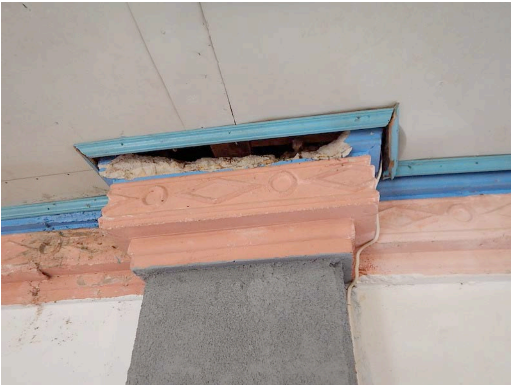
Figure 60. The interior pilaster or concrete capital shows damage of its top molding, possibly from seismic movement of the ceiling, or during the ceiling reinstallation.
