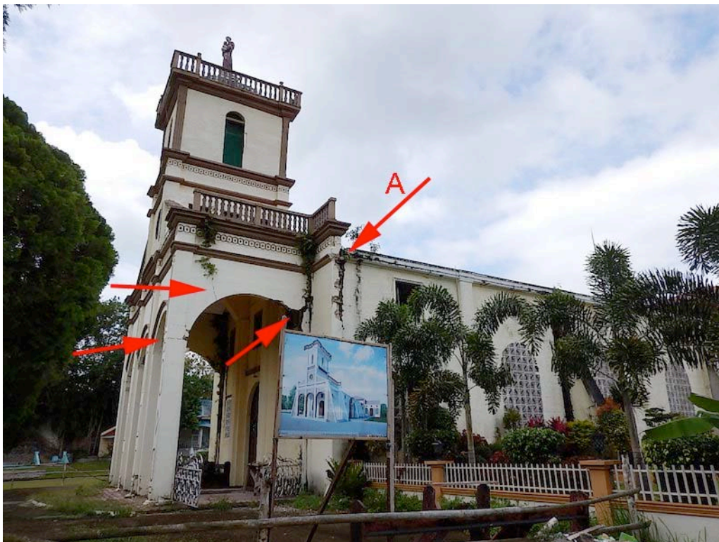
Figure 46. View of east side of the portico and bell tower, with the arrows pointing to crack, which all appear to be from rocking of the bell tower and portico. See fig. 58 for interior view of the crack at "A."
