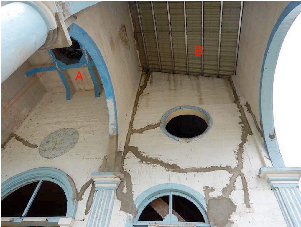
Figure 33. Facade and underside of portico, showing recently patched concrete, which is recommended to be monitored for durability. At the central bay at “A” can be seen the framing for the floor of the bell tower, which has haunches where the beams meet the walls, and diagonals in the corners, both modern concrete details designed to resist rocking and twisting during earthquakes. At “B” is the underside of the roof, which indicates that the two outer bays of the portico are less rigid and can twist during an earthquake.
