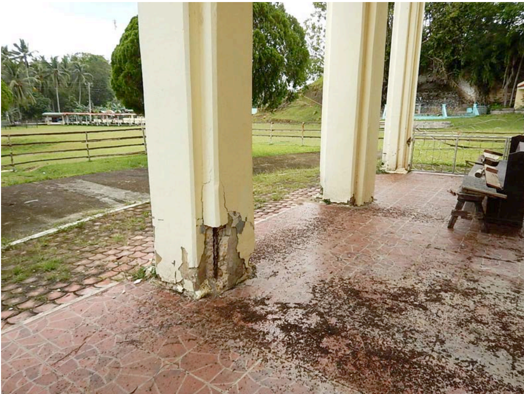
Figure 54. Concrete portico columns are typically cracked and spalled at the bases from bending. This is a common damage type for portico rocking caused by a soft-story and mass irregularity such as a bell tower.
