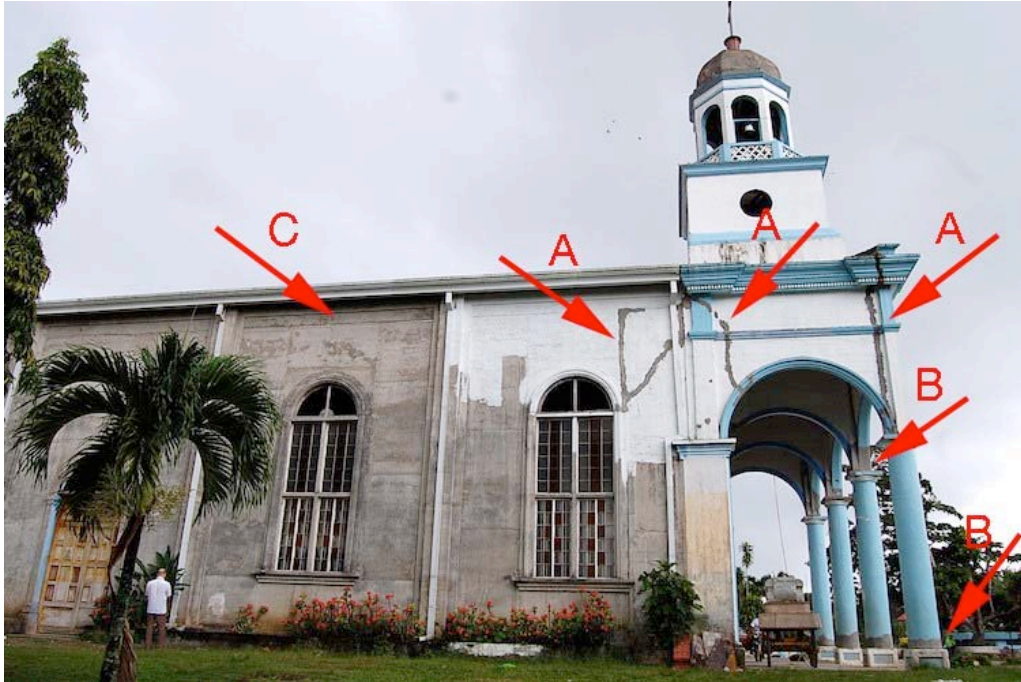
Figure 32. View of the south side of the portico and bell tower and partial south elevation. The cracks at “A” and “B” match those in the previous figure. At “C” can be seen what appears to be a beam connecting the tops of the frame columns. See interior view of beam in fig. 43.
