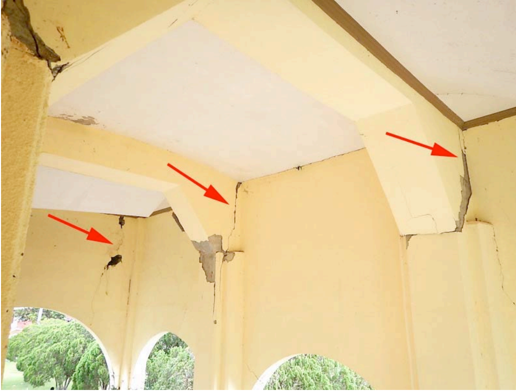
Figure 53. View beneath the portico. Note the cracks around the beam haunches from rocking of the portico and bell tower.
