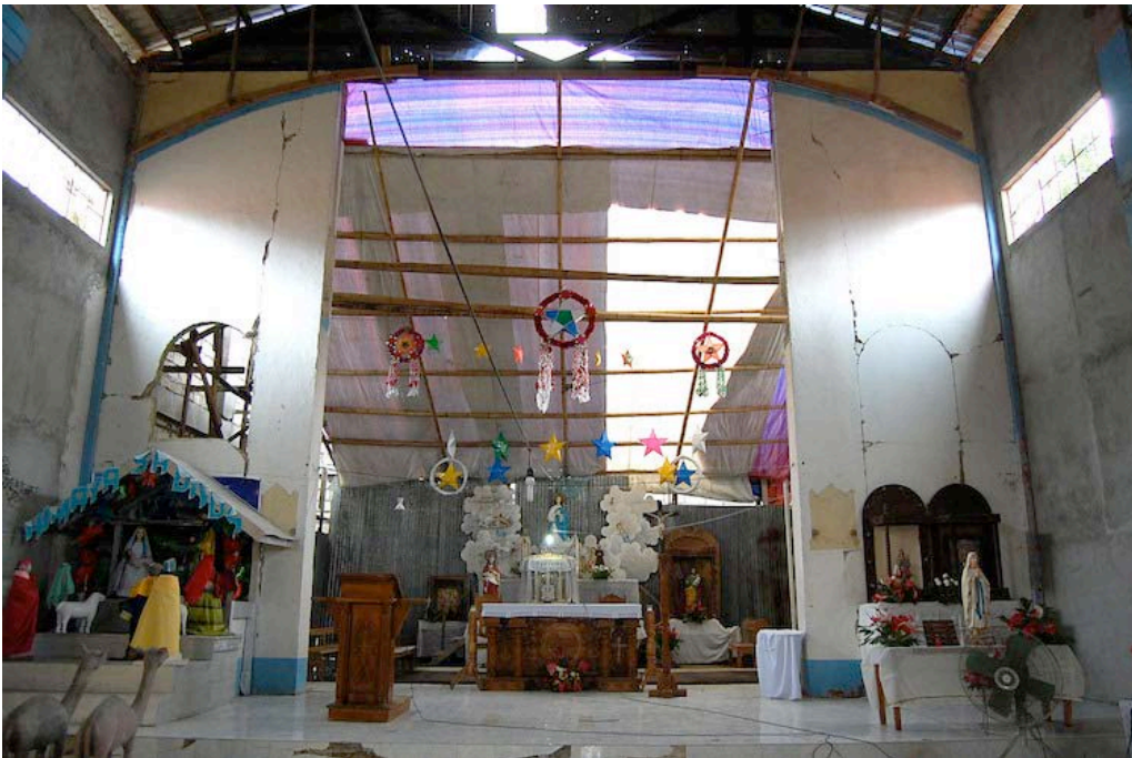
Figure 41. View of the altar, showing cracks and collapsed sections.
