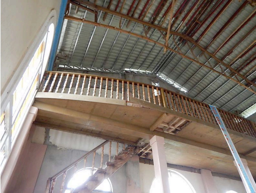
Figure 42. View of the choir loft. Note missing plywood panel ceilings, and steel roof purlins in one section of the roof.
