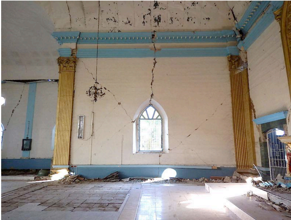
Figure 25. View of the north nave wall on the east side of the transept, showing damage similar to the other section of the north wall in fig. 23.
