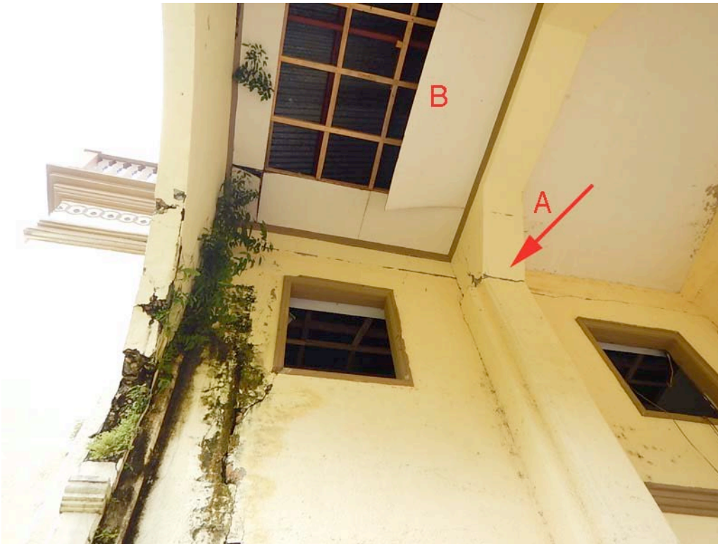
Figure 52. View of the front facade at the southwest corner. Note cracked concrete at haunch at “A,” and fallen ceiling sections at “B.” The roofing can be seen above the ceiling, indicating that the portico structure is similar to Catigbian (see fig. 33), so prone to twisting during an earthquake.
