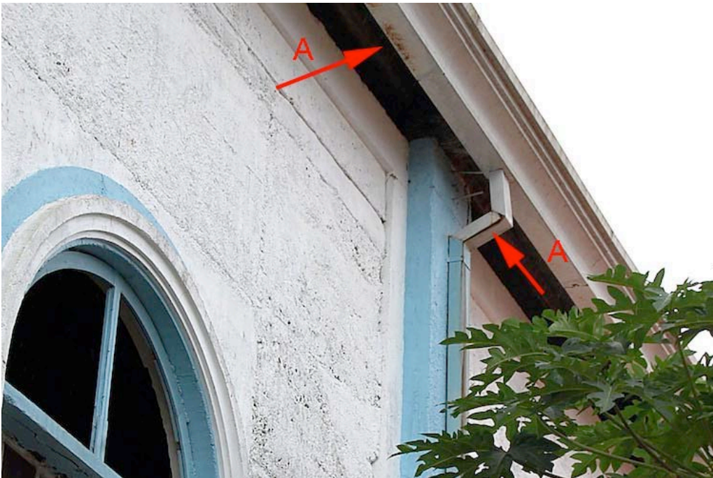
Figure 37. Underside of the metal gutters, showing rusting, and open joints and rusting of the downspouts.
