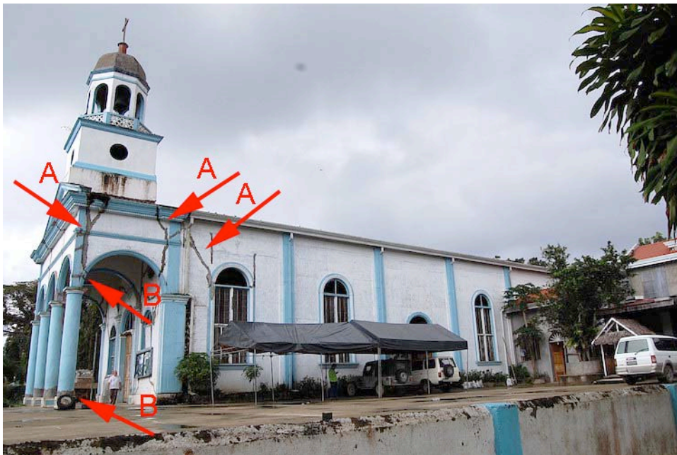
Figure 31. View of the north side of the portico and bell tower and north elevation. The cracks at “A” appear to be from rocking of the portico and bell tower from soft-story and mass irregularities. The cracks at “B” are from bending of the columns during the portico rocking motion.
