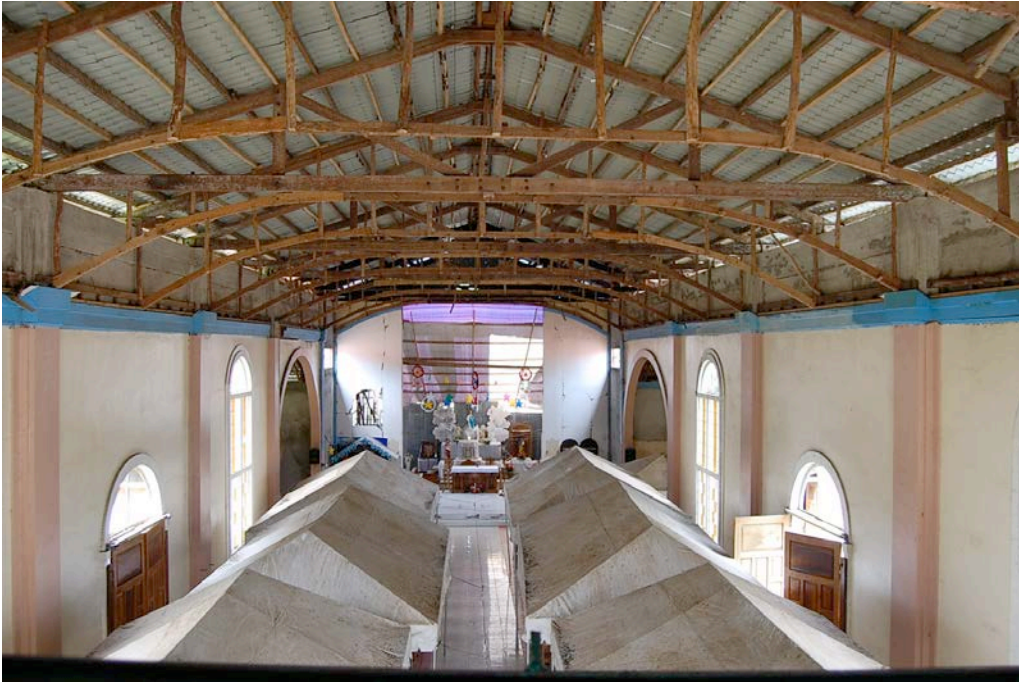
Figure 40. View from balcony looking towards the altar. Note the missing finished ceiling, exposing the lightly framed roof structure.
