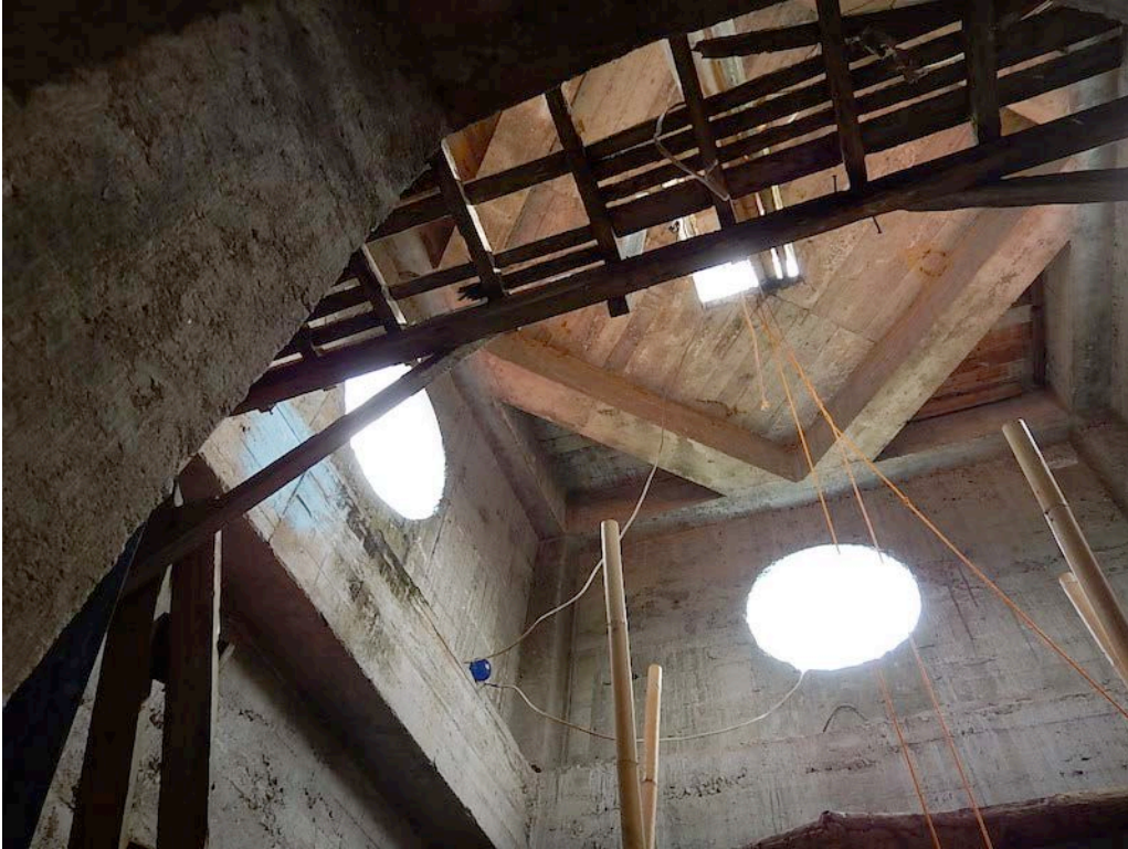
Figure 34. Interior view of the bell tower, underside of portico, showing the diagonal beams in the floor framing, which are designed to resist twisting during earthquakes.
