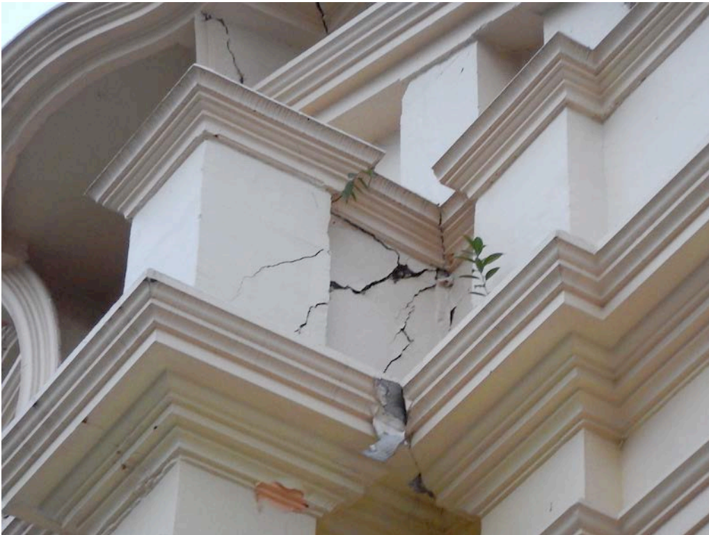
Figure 12. Another view of the pediment over the front facade showing diagonal cracks in the concrete, probably from rocking of the pediment.
