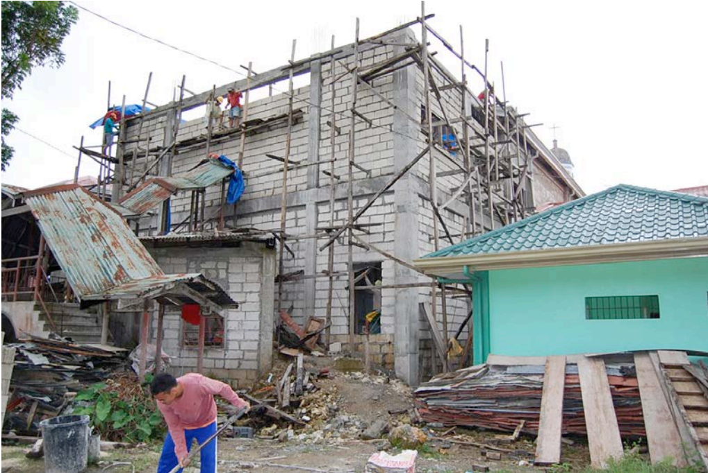
Figure 36. Addition to the west end of the church, using what appears to be confined masonry type of construction, which is designed to be resistant to earthquake motion, by the use of a full concrete frame, with columns connected at the top and floor levels with beams, and infilled with unreinforced concrete block.
