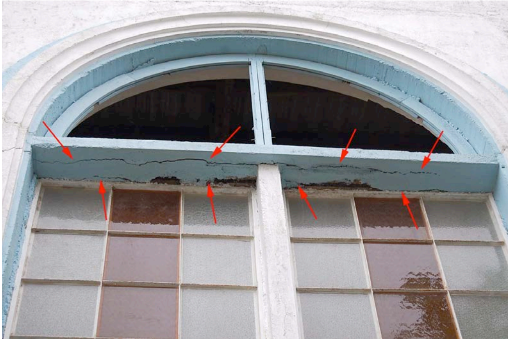
Figure 38. Typical view of steel casement windows with colored glass. The arrows point to cracks in the concrete transom bar, probably caused by rusting steel reinforcing bars, which is not seismic damage.
